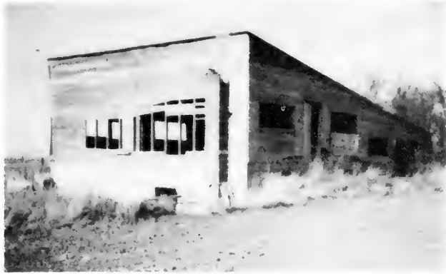
This deteriorating warehouse is all that is left of the once thriving Kruger orchard.
